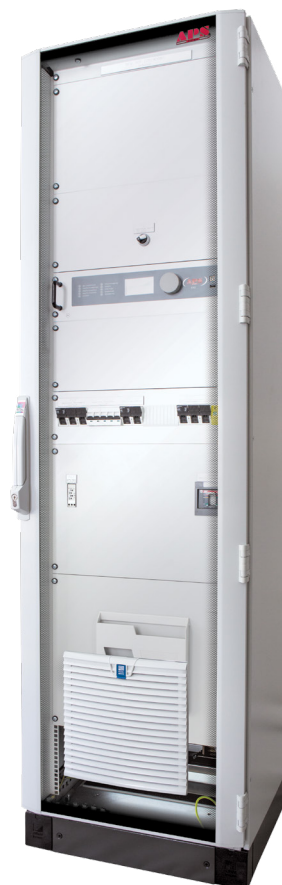
View of the non-transformer UPS cabinet
