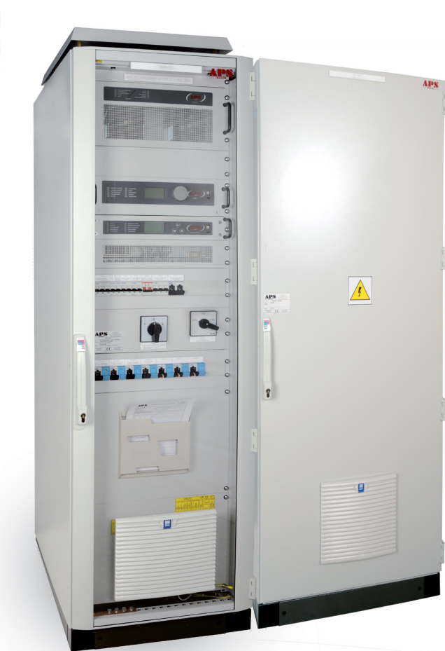
View of the UPS system cabinet
