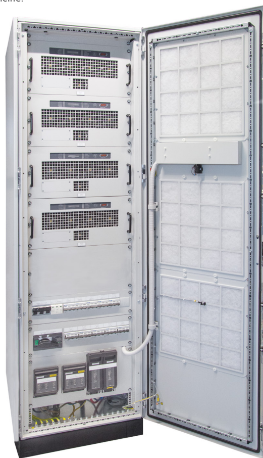
View of the non-transformer UPS cabinet
