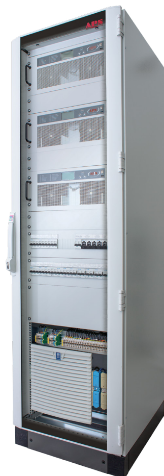
Views of the rectifier cabinet
